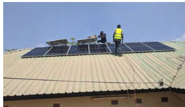
WHO and Prudential supported Health Facility Solarization at Chalimbana Health Centre, Chongwe District, August 2025
