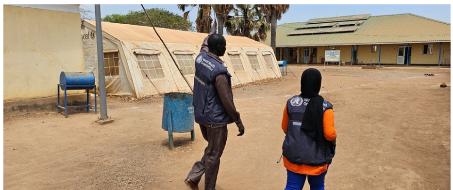
Improvised tent for a CTU at Kuajok hospital that was advised to be dismantled because of inappropriate location following technical assessment
