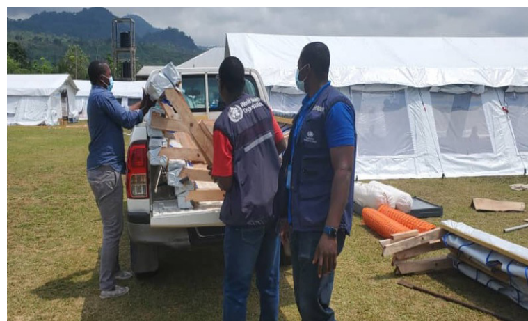
Unloading the building material for the marquees to extend the hospital capacity of the CDC hospital in Bota, Limbé in the South-West, in November 2021.
