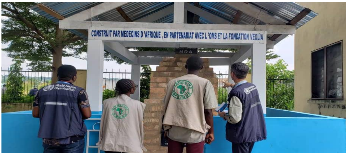
To ease the destruction of hazardous biomedical waste, WHO partnered with @FondationVeolia, @medecin-afrique to construct a biomedical waste incinerator at the M'filou hospital in Brazzaville/WHO-Marriane Tabi
