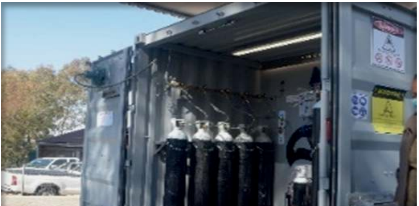
Oxygen plant at the Berea Hospital
