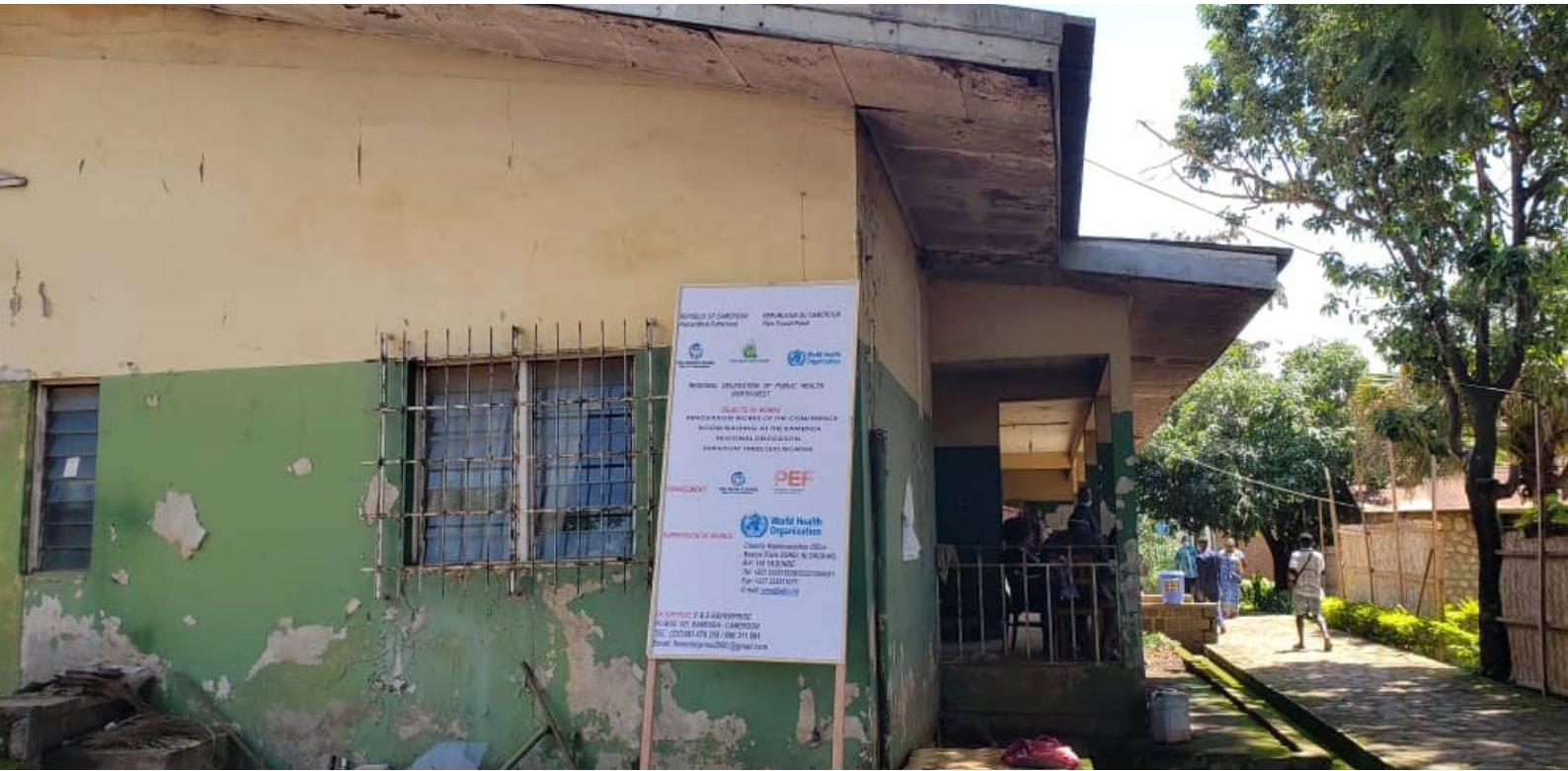
Photo : The Public Health Emergency Operations Centre (PHEOC) of Bamenda, before renovation
