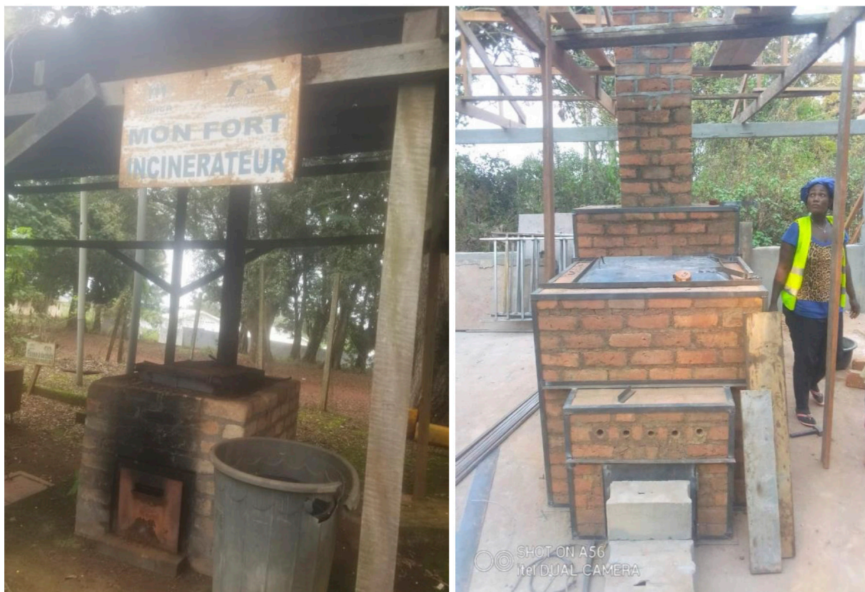
Old and new incinerator under construction in Batouri Health District, Eastern Region
