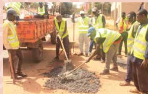
Road workers from the National Roads Authority mending potholes in Bakau town
